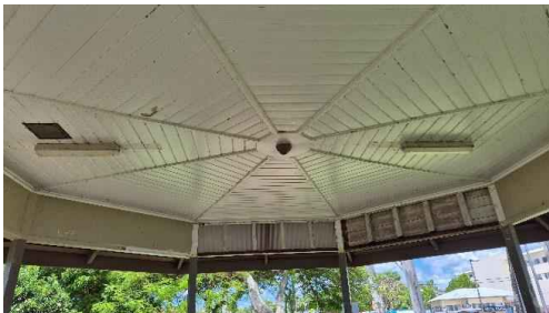
Figure 26: Ceiling showing two lights and a manhole cover. Also note the upper panel with missing sections.
